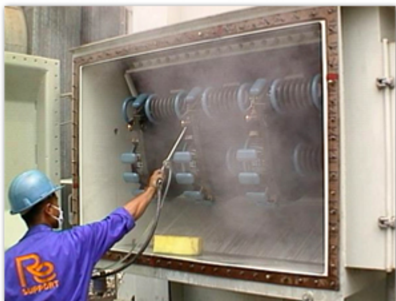
"ABB" on Load Tap Changer Inspection, Oil Replacing and Overhauling
