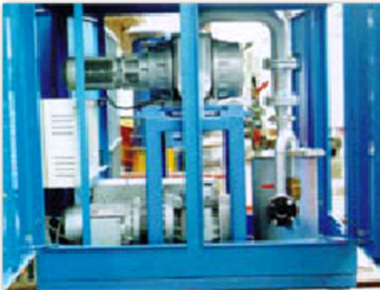
"Rietschle-Germany" 14000 Litre/Minute Rotary Vane Vacuum Pump Combination with Roots Pump
