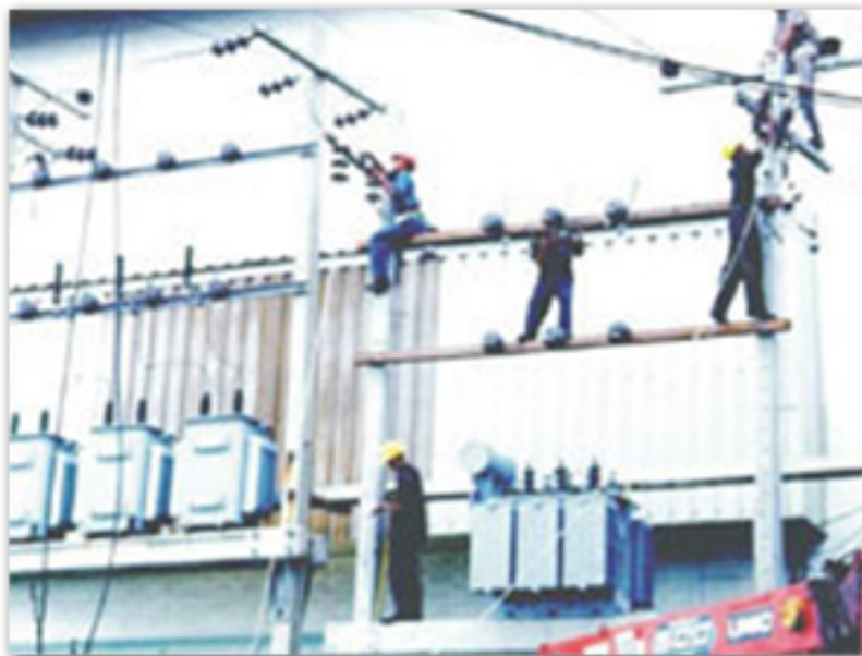
High Voltage Cleaning and Preventive Maintenance
