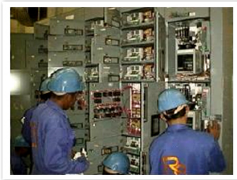
“Switchboard” Preventive Maintenance
